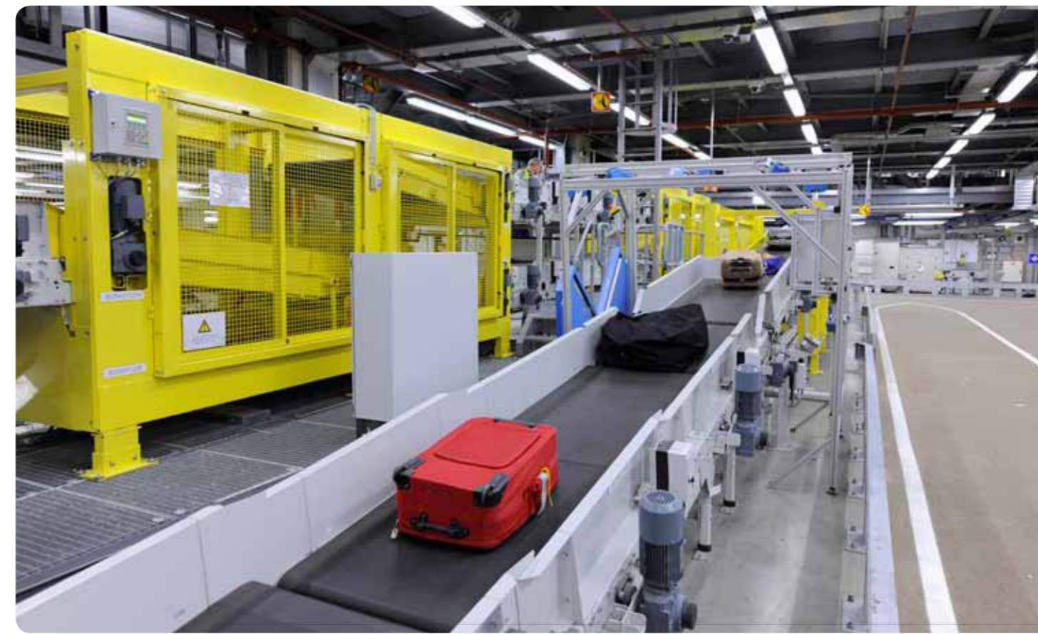
The baggage basements house 21 kilometres of conveyors and a five-kilometre rail system. Schiphol has the most advanced baggage system in the world.
